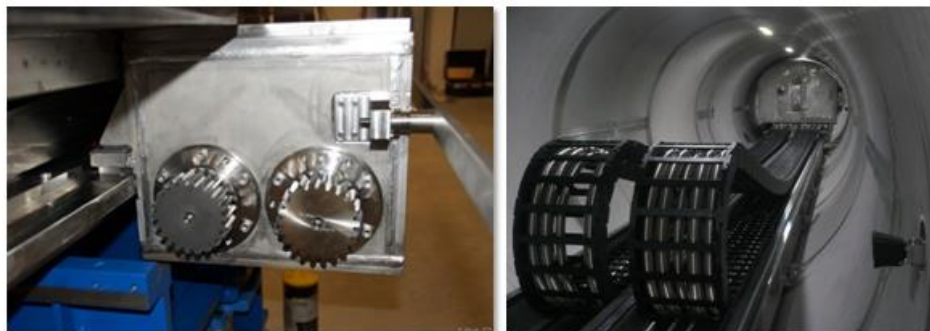
Figure 7 a and b: (a) Double pinion of the motor box. (b) Flexible corrugated tubes inside two cable chains.
